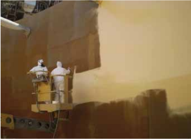
ABOVE ▲ The crew used a Graco 74:1 spray pump to spray-apply the specified two coats of Carboline 235 at 6-8 mils (0.15mm-0.20mm) DFT per coat.
