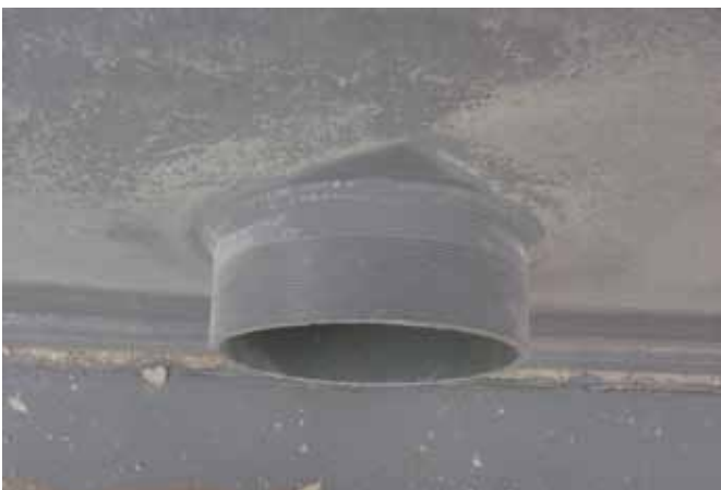
BELOW ▼ After one year of hard service, even the 8" (20.32cm) threaded pipe nipple was rust-free.
