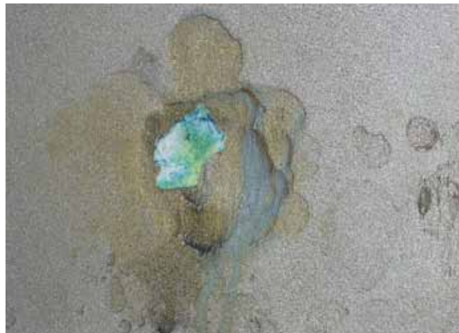
ABOVE ▲ "Then he [Brodar] got some yellow paper and a spray bottle. Every place he sprayed with distilled water and applied the paper changed color from yellow to blue. He explained that it was an indicator of chloride contamination on the steel," says Carlisle.
