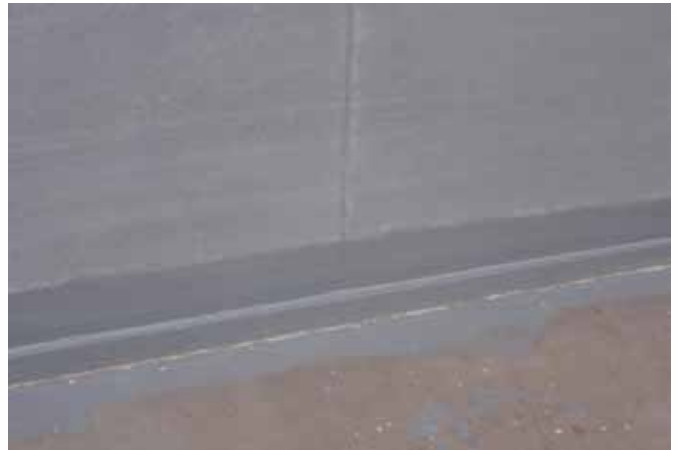
ABOVE ▲ Even at the steel/concrete interface there were no signs of corrosion upon inspection after one year in immersion service.
