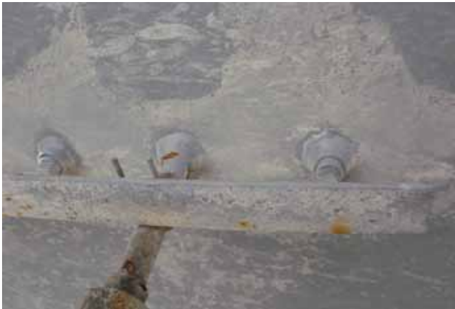
ABOVE ▲ At the year-anniversary inspection, the only rust observed on the carbon steel substrate was observed on this pipe.
