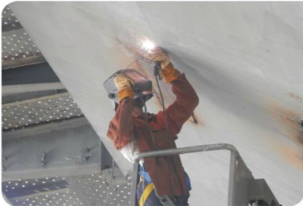
The crew worked from a barge with a 2-ton (1.8 metric tons) man lift. Even with the lift, getting access to all of the nooks and crannies on an angled surface has been a challenge.
