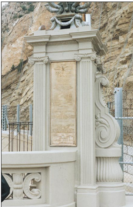
Pylon and plaque four years after repairing, cleaning, including soluble salt removal, and coating
