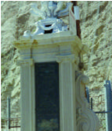
Top: Pylon before rehabilitation in 1995. Center and bottom: Pylon in September 2004. There is minor rust staining from the fixture above. Completely intact as completed in 1995 with some small rust stain bleeding from above.
