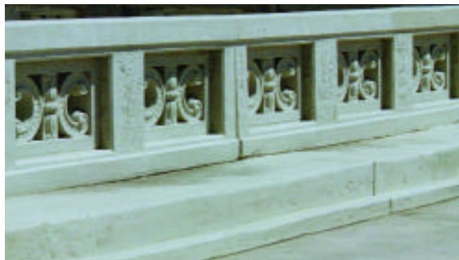
This sidewalk area has had puddled standing water since being repaired and recoated but the coating remains intact Photos courtesy of Chlor*Rid
